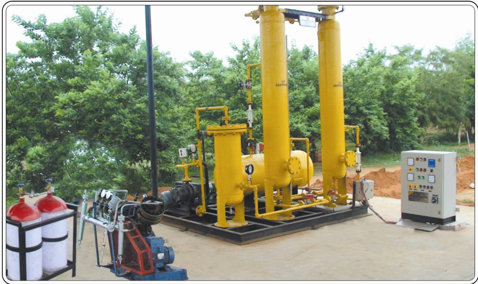
VPSA System with 2 stage compressor, Control Panel & CBG Cylinders
